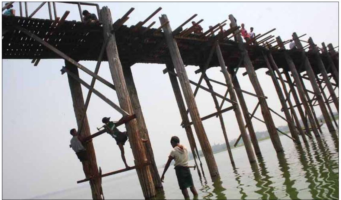
Workers repair sections of U Bein Bridge in Amarapura township in March 2014. Photo: Phyo Wai Kyaw
