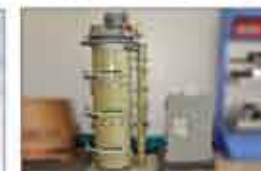
On Load Tap Changer (M/S, Germany)
