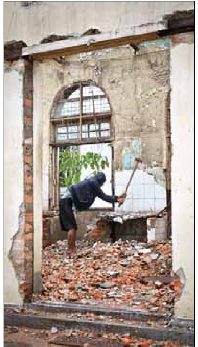
A worker deconstructs the building at 233-235 Pansodan Street in October, before demolition was halted following a media campaign by heritage activists. Pic: Boothee
