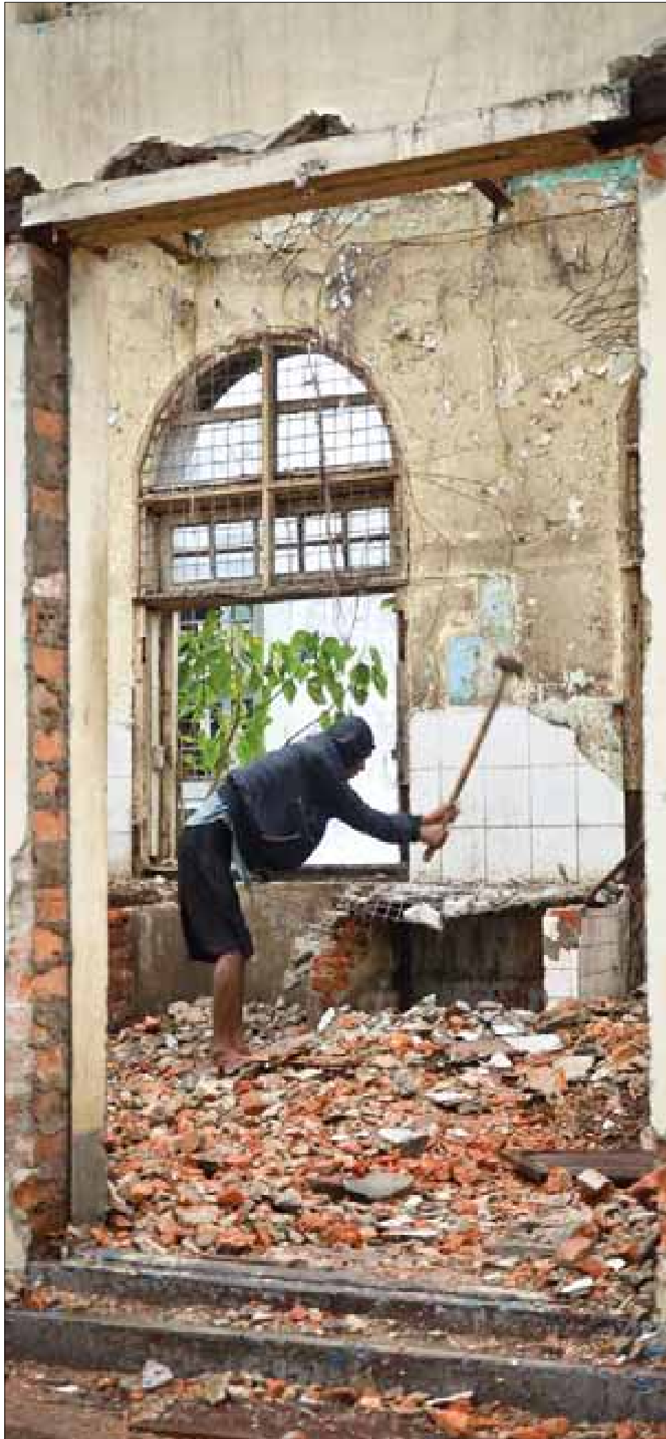
More page 4 A worker destroys sections of the upper floor of 233-235 Pansodan Road. Pic: Boothee
