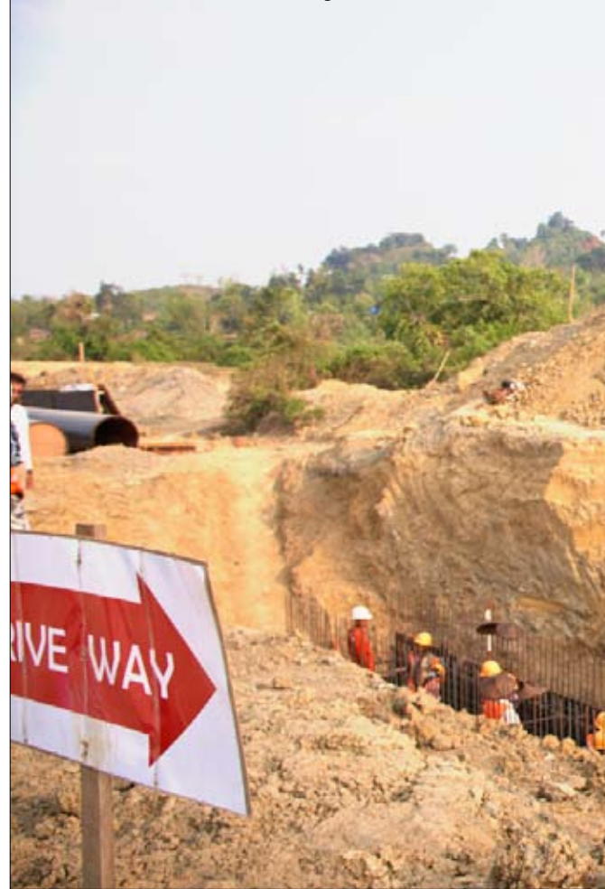
A worksite for the Myanmar-China oil and gas pipeline in Kyaukpyu township, Rakhine State. Pic: Juliet Shwe Gaung
