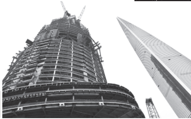
The foundation for the world's second tallest building has been completed in Shanghai, on 27 Dec, 2011.—XINHUA
