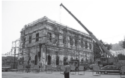
Egyptian workers repair the building of Scientific Institute in Cairo, Egypt, on 27 Dec, 2011. The Scientific Institute was built in 1798. XINHUA
