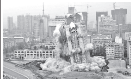
An office building of local government is demolished in directional blasting in Kunming, capital of southwest China's Yunnan Province, on 25 Dec, 2011. After the directional blasting, a business center will be constructed in the area. The new office building of Kunming municipal government will be built in a new district of the city.—XINHUA
