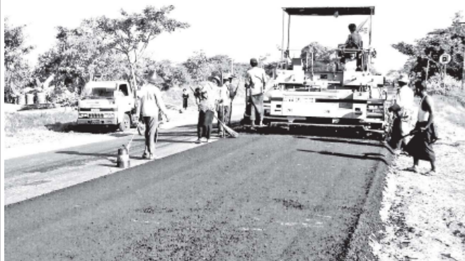
Bago-Nyaunglebin section of Yangon-Mandalay Union Highway being upgraded with asphalt concrete by Shwe Than Lwin Co through BOT system.
