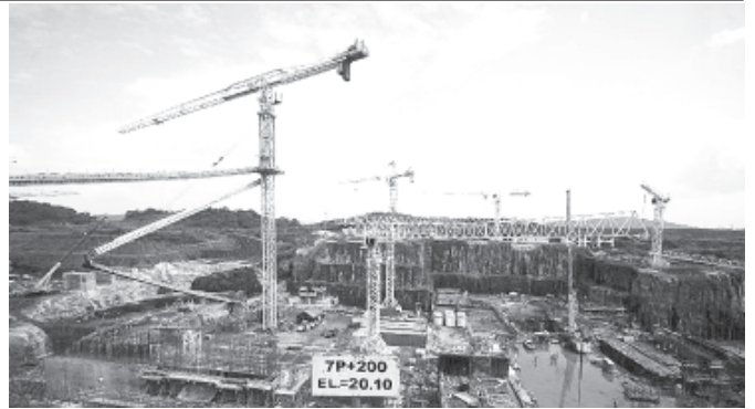
Machines work at a construction site in Panama Canal, Panama, on 21 Dec, 2011. The canal expansion is expected to be completed by 2014, the waterway’s 100 th Anniversary.—XINHUA
