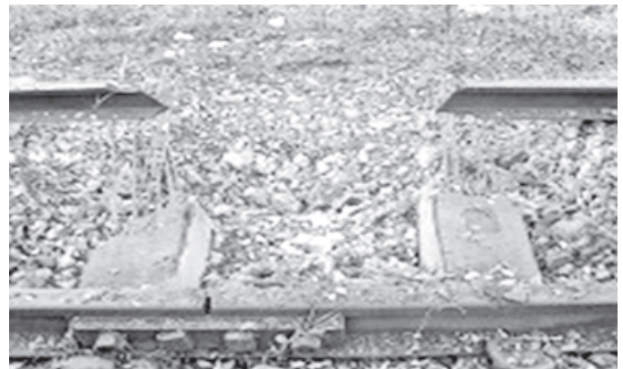
Damaged railway joint seen between milepost Nos 678/11 and 678/14 due to a series of blast between Htopu and Hsahmaw stations.—MNA
