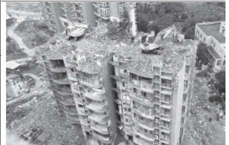
Photo taken on 6 Dec, 2011 shows mechanical diggers dismantling a tottering "risky residential building" in Yuhuan County of Taizhou City, east China's Zhejiang Province. The building, delivered last January, inclined west on the afternoon of 1 Nov due to a weak pile foundation.—XINHUA
