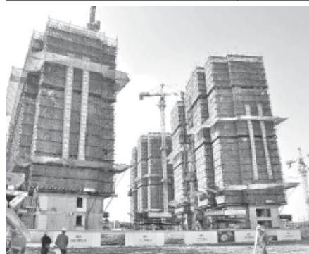
Photo taken on 27 Nov, 2011 shows the construction site of an indemnificatory housing project in Baoshan District of Shanghai, east China. The launching goal of Shanghai's indemnificatory housing construction is expected to be achieved at the end of November. About 170,000 indemnificatory housing units are scheduled to be provided to low-income families in 2011.
