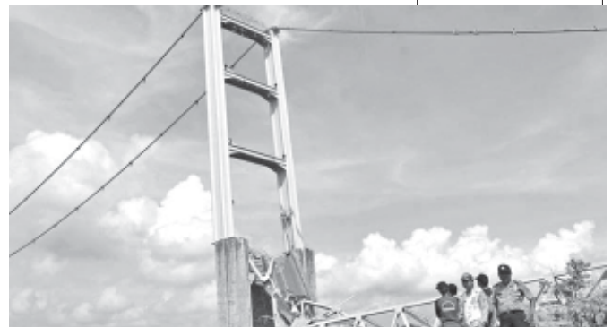
Rescuers inspect the ruin of Kutai Kartanegara bridge in Tenggarong, East Kalimantan, Indonesia. INTERNET
