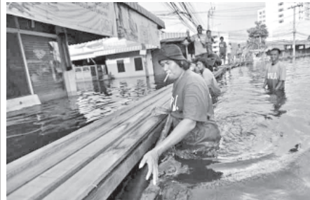
Workers from Bangkok Metropolitan Administration construct a temporary walkway over floodwaters at a neighbourhood in Bangkok, Thailand.—INTERNET
