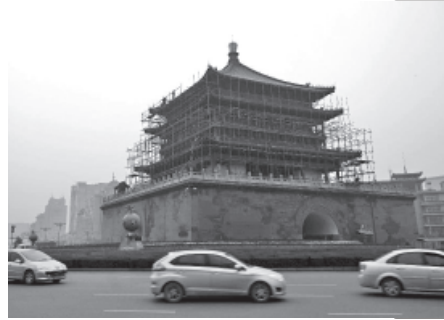
Photo taken on 16 Nov, 2011 shows the Bell Tower under maintenance, in Xi'an, capital of northwest China's Shaanxi Province. The Bell Tower, built over 600 years ago in Ming Dynasty (1368-1644), closed temporarily to tourists for routine maintenance.—XINHUA
