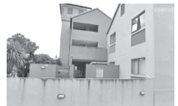
The 32 units of the Pepperwood Mews apartment complex were emptied of all their fixtures and fittings.— INTERNET
