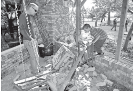
Jess Burrow, left, and James Patterson, look over the damage caused outside the home of Joe and Mary Reneau when their chimney was toppled by Saturday's earthquake, in Sparks, Okla, on 6 Nov, 2011.
