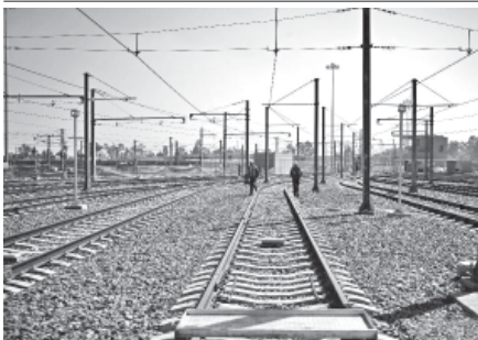
Workers walk on the tracks of the new subway line in Mexico City, capital of Mexico, on Nov. 1, 2011. Line 12 is on its last construction stage and the tests are underway, it will link the west and the east side of the metropolis. The line is expected to begin operation next April.—XINHUA
