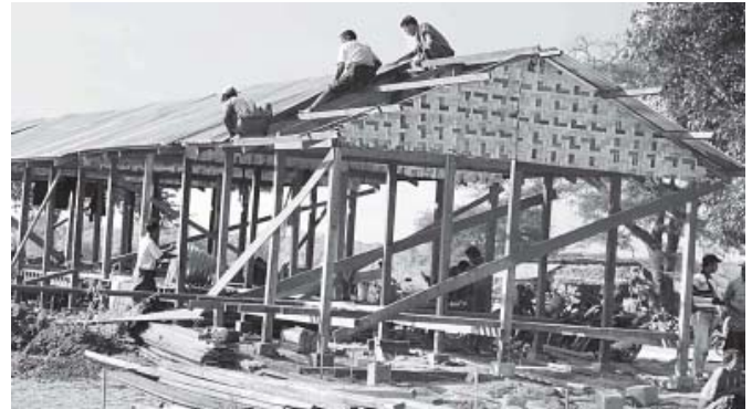
Tatmadawmen building houses at Sunthike Ywathit field in Kywete Village-tract in Pakokku Township.—MNA
