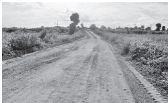
Ministry of Border Affairs repairing roads in Seikpyu Township of Pakokku District.
