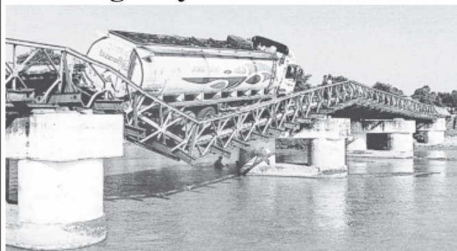
Watkot Bridge across Taungyama Creek seen collapsed after an overloaded vehicle has passed on it.—MNA
