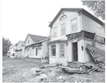
Flood-damaged houses line the main street in Prattsville, NY, on 12 Oct, 2011. Tropical storms Irene and Lee have left its victims tired and frustrated more than a month after the back-to-back disasters swamped homes, washed away roads and upended life in a region not accustomed to massive flooding.
