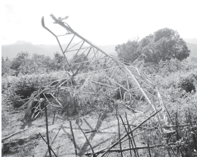
Suspension Tower No. SM-129 of 230 KV Shweli-Mansan power grid blasted by insurgents.
