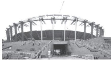
Workers carry out reconstruction operations at the Olympiysky stadium in Kiev, May 2011.— INTERNET
