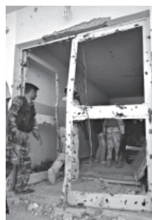
Iraqi security forces inspect the damaged at a police station in al-Baghdadi west of Ramadi, 70 miles (115 kilometers) west of Baghdad, Iraq, on 3 Oct, 2011.
