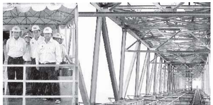
Deputy Minister for Construction U Kyaw Lwin inspected construction of Ayeyawady Bridge (Pakokku) on 2 October. (News reported)—MNA
