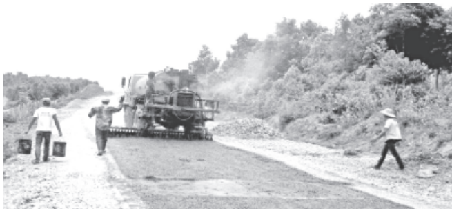
Tarmacking work in progress with the use of heavy machinery on PyinOoLwin-Mogok road.
