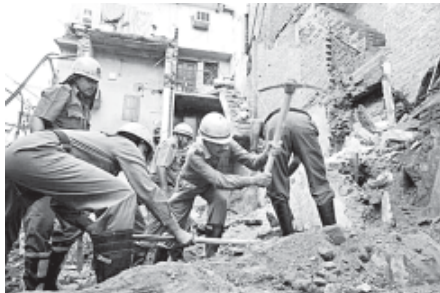
Indian rescue workers dig the rubble from the decades-old building that fell Tuesday night in the Old Delhi area of New Delhi, India, on 28 Sept, 2011.—INTERNET
