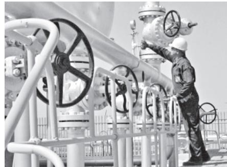
In this Tuesday, 15 April, 2008 file photo Iranian oil technician Majid Afshari checks the oil separator facilities in Azadegan oil field, near Ahvaz, Iran.—INTERNET
