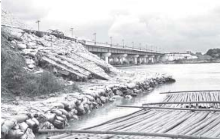
Photo shows preventive measures against erosion at Swa Creek Bridge on Thagara-Myochaung section of Yangon-Mandalay Expressway. Ko Lwin-Swa
