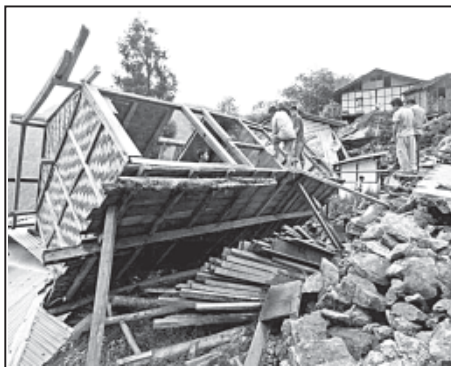
People repair their house damaged in Sunday's 6.9-magnitude earthquake in north of Gangtok, India, on 21 Sept, 2011. Indian soldiers managed to reach a hydroelectric project in the northeastern Wednesday where many people were killed in a series of landslides triggered by a powerful earthquake. INTERNET
