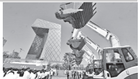
Photo taken on 19 Sept, 2011 shows the ceremony for the beginning of the construction of the city's tallest skyscraper in Beijing, capital of China. Beijing will begin building the city's tallest skyscraper in its central business district.—INTERNET
