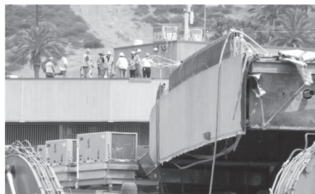
Border officials and emergency personnel look over the construction site where a scaffolding collapsed at the San Ysidro Port of Entry in San Diego on 14 Sept, 2011.—INTERNET
