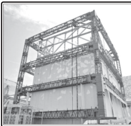
Steel frame constructed for the cover of Tokyo Electric Power Co (TEPCO)'s Fukushima Daiichi Nuclear Power Plant's Unit 1 reactor is completed in this handout photo taken by TEPCO in Fukushima Prefecture, northern Japan, on 9 September, 2011 and released on 10 September, 2011. INTERNET
