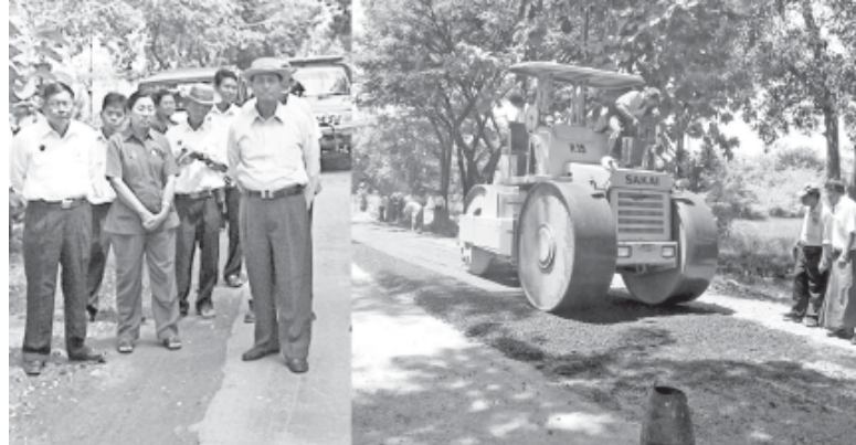
Union Minister for Construction U Khin Maung Myint inspects repaving of Yangon-Pyay Road between milepost Nos. 93/4 and 93/5. MNA
