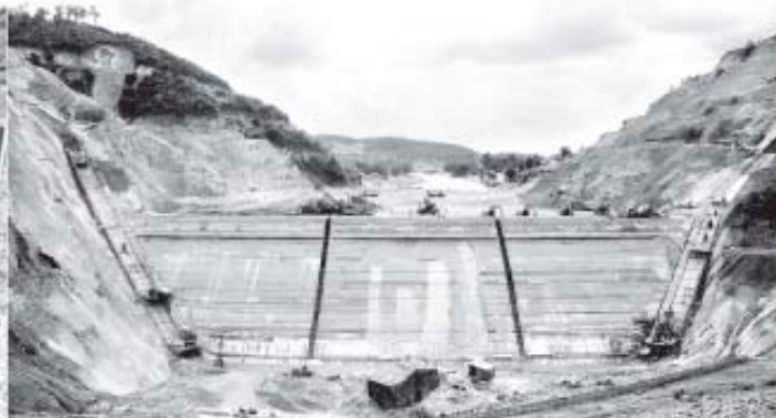
Vice-President Thiha Thura U Tin Aung Myint Oo views progress in implementing Thaukyekhat -2 Hydropower Project. MNA
