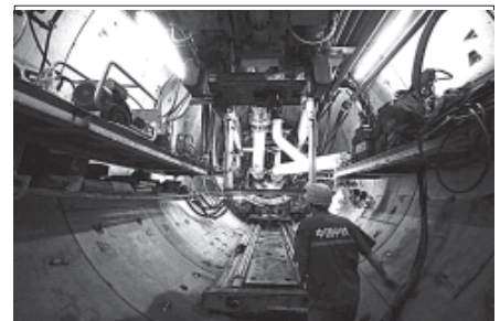
A worker walks towards the tunneling machine used in the subway construction under the Yangtze River in Wuhan, capital of central China's Hubei Province, on 21 Aug, 2011. XINHUA
