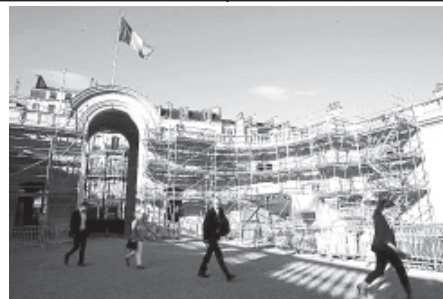
People walk in front of the Elysee Presidential Palace under renovation in Paris, France, on 16 Aug, 2011. The Elysee Palace is receiving renovation during the summer vacation of August. The restored Palace will be accessible to public in the upcoming European Heritage Days on 17 Sep and 18 Sep, 2011. XINHUA
