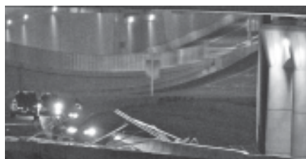
Part of the 17th Street bridge that spans Atlanta's downtown connector collapsed onto the northbound lanes of Interstate 85 before midnight on on 13 Aug, 2011, causing large traffic delays in the midtown area of Atlanta. INTERNET
