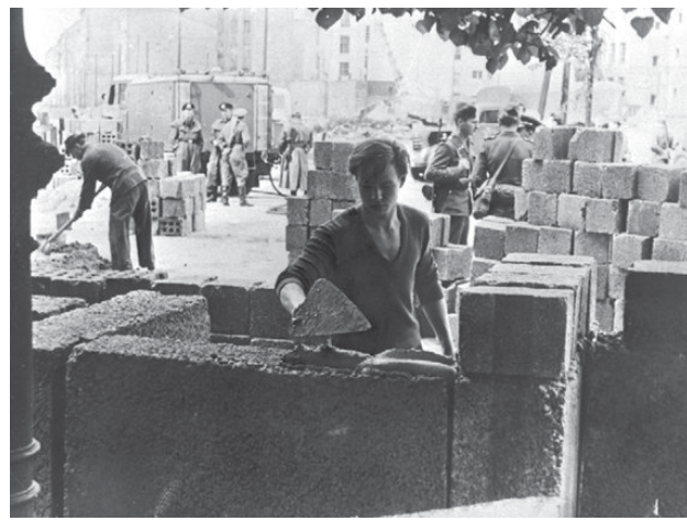
In this 13 Aug, 1961 file photo a worker builds parts of the a wall between the eastern and the western part of Berlin. AP Photographer Peter Hillebrecht was on assignment in Berlin as the construction of the Berlin Wall starts on 13 Aug, 1961 and he was one of the first photographers to cover this historic event. INTERNET
