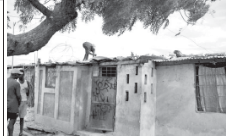
A man makes repairs to his roof in the shanty town slum area of Cite Soleil on 4 Aug, 2011.
