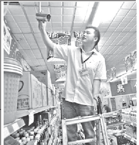
A worker checks a camera in a supermarket in Huixinli, Chaoyang District, Beijing on Monday. The public security bureau has ordered high-fidelity monitoring devices to be installed in large and medium-sized supermarkets across the city for security reasons.— INTERNET
