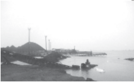
Image of the collapse of a section of the dock of bridge Ibicuy, located in the province of Entre Rios, Argentina, on 18 July, 2011. XINHUA
