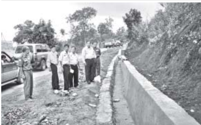
ROAD WORKS INSPECTED: Deputy Minister for Construction U Soe Tint made an inspection tour of Pyay-Paukhaung-Ottwin-Toungoo Road on 11 July. He looked into construction of retaining walls for proper flow of water along the road as part of efforts to maintain road sections in rainy season.—MNA
