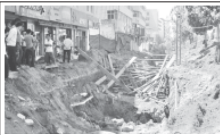
Photo taken on 10 July, 2011 shows the collapsed framework at a construction site for replacing heating pipelines in Ongniud Qi of Chifeng City, north China's Inner Mongolia Autonomous Region.—XINHUA
