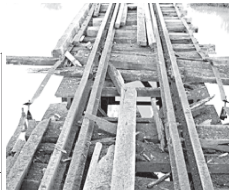
Photo shows destructions on the rail tracks between Hopin and Nankhwin of Mandalay-Myitkyina railroad due to mine blast planted by KIA group.
