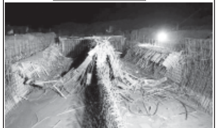
Photo taken on 29 June, 2011 shows the collapsed tunnel in an under-construction airport in Kunming, capital of southwest China’s Yunnan Province.—XINHUA
