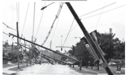
A row of electric power poles snapped along Floyd Street at Central Avenue in front of Cardinal Stadium at the University of Louisville in Louisville, Ky, on 22 June, 2011 after an apparent tornado moved through the area.
