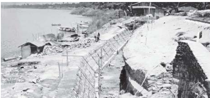
The Directorate of Water Resources and Improvement of River Systems is building a concrete embankment along the bank.
