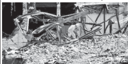
Photo taken on 19 June, 2011 shows the steel structure collapse site in Heshan Electricity Generating Company in Heshan City, south China’s Guangxi Zhuang Autonomous Region.—XINHUA
