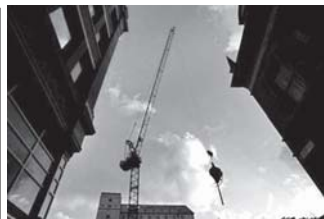
A construction crane at a building site in central London. The International Monetary Fund said there is danger the fragile global recovery could collapse unless Europe averts sovereign defaults, the United States gets its fiscal house in order and emerging economies prevent overheating.—INTERNET
