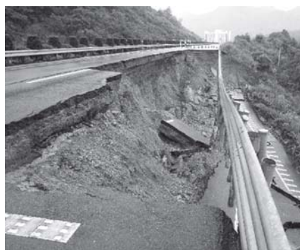
Photo taken on 15 June, 2011 shows road surface of Hangxinjing Highway caves in Hangzhou, capital of east China's Zhejiang Province. The collapse extends 80 meters with width of 7-8 metres, forcing the highway to close. No casualties were reported.—XINHUA
