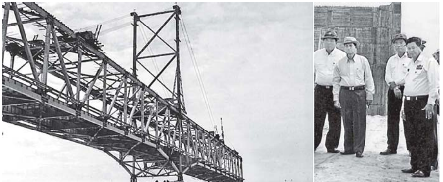
Union Minister for Construction U Khin Maung Myint inspects installation of steel truss of Ayeyawady Bridge (Nyaungdon).—MNA
