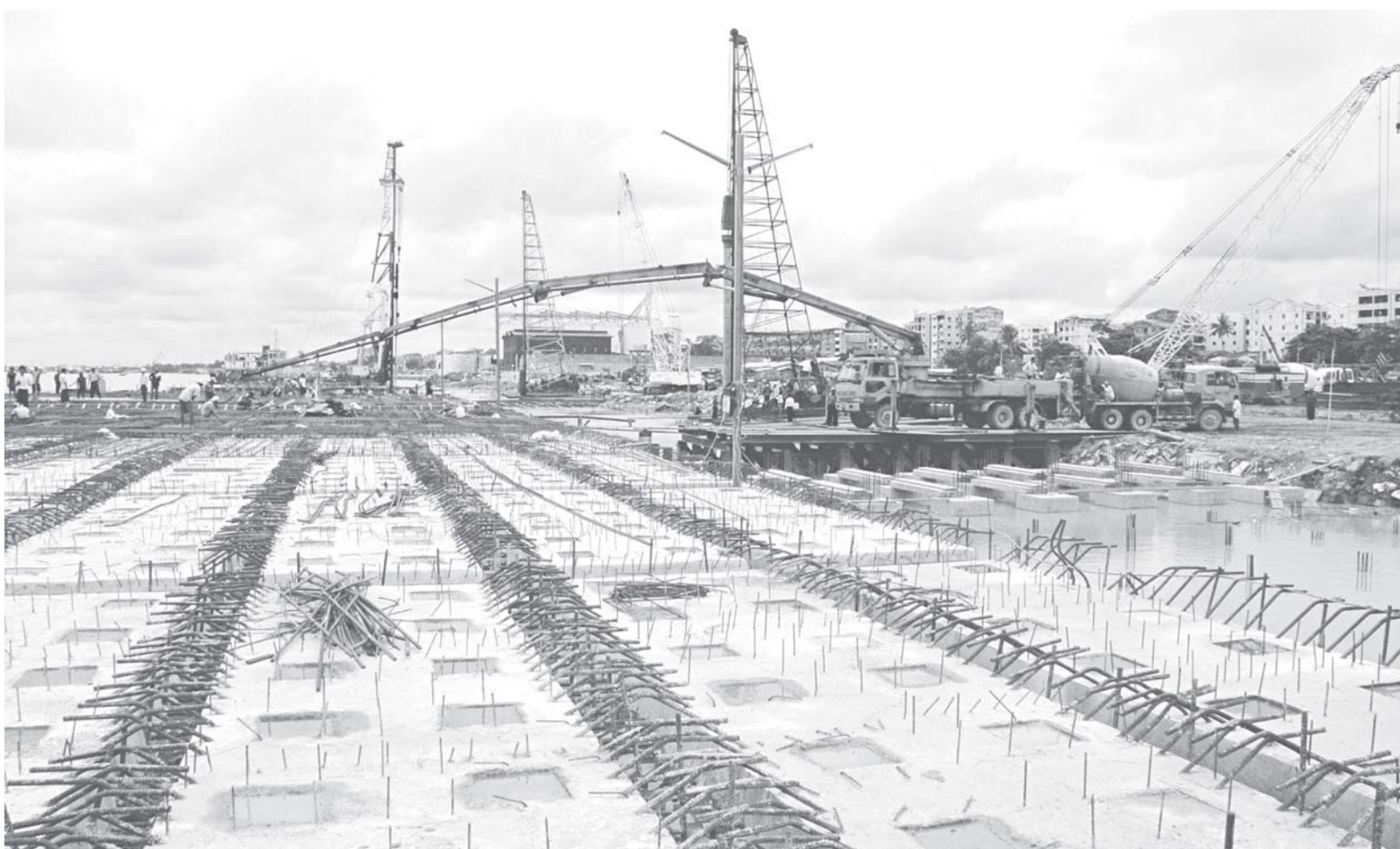
Photo shows Asia World Jetty which is under construction for extension in Ahlon Township.—MNA
