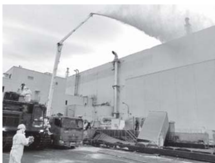
Handout photo issued by TEPCO shows workers spraying a dust inhibitor into buildings at the firm's crippled Fukushima nuclear power plant. Japan has more than doubled its initial estimate of radiation released from the nuclear plant in the week after the 11 March tsunami, ahead of the launch of an official probe Tuesday.
